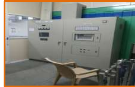
VHT CONTROL PANEL
